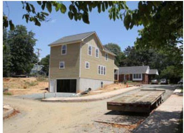
Francis Fife Way contains new homes being built by Habitat for Humanity.
