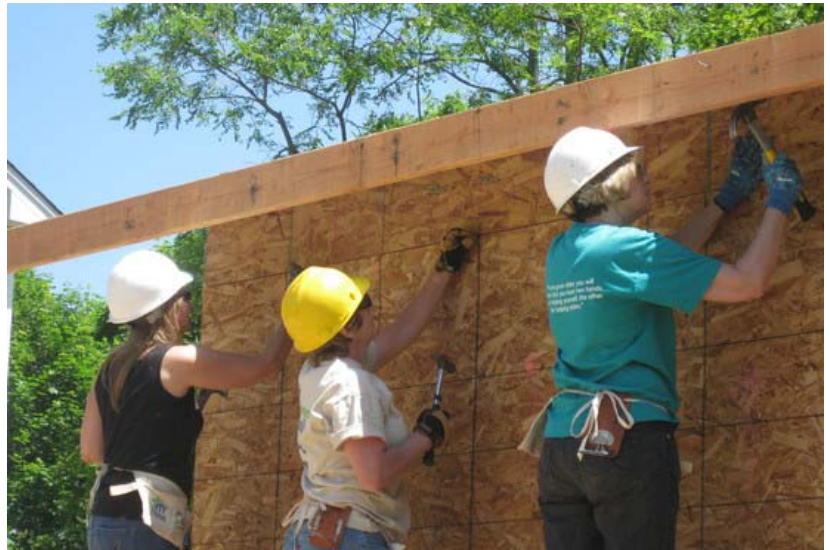
Dawn Wotapka/The Wall Street Journal Habitat for Humanity volunteers help build the home of Cheri Sabolenko in East Patchogue, N.Y., in May.
